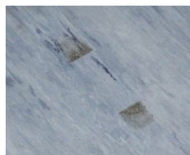
Discolouration and imprints due to unsuitable castors
