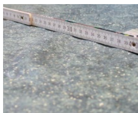
Irreparable damage caused by hard castors
