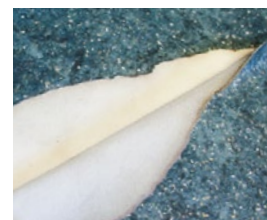
Delamination after overloading by chair castors
